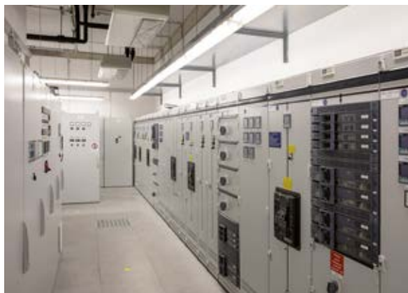
All processes at the Grüneck wastewater treatment plant are largely digitalised.
