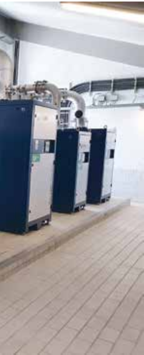
Five turbo blowers from AERZEN ensure the oxygen supply in the aeration tanks.
