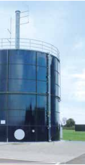
The gas storage tank has a capacity of approx. 500 m 3 .
